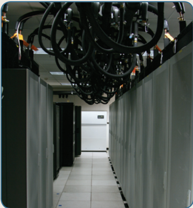
Each computer rack is cooled by a closed-loop chilling system. Photo by Nile Mueller.
